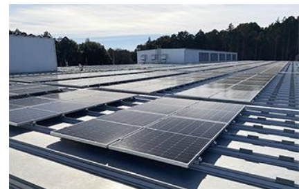
The solar system at Shiroy Data Center Campus
